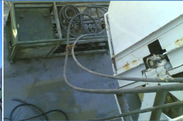
Power unit that feeds the power tong
